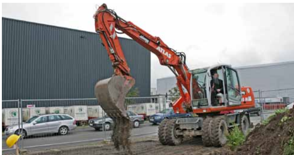
A size larger: Frank Benzinger, manager of vhf camufacture AG, digging with the excavator the first bit of the building pit of the project
