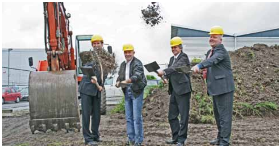
With vim and vigor at the ground-breaking ceremony (from the left): Friedrich von Ow-Wachendorf, mayor of Ammerbuch, Wolfgang Gsell, chairman of the vhf supervisory board, Jaromir Bednarik, general building contractor and Frank Benzinger, manager of vhf camufacture AG.
